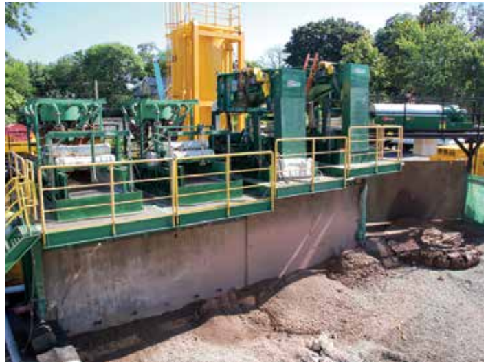
Derrick Modular Slurry Separation Plant and DE-7200 VFD Centrifuge
