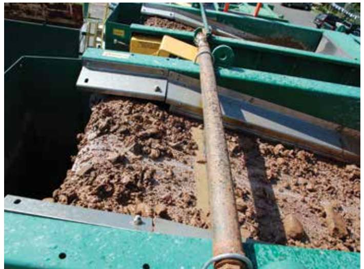
Two Derrick Flo-Line Primers handling primary separation
