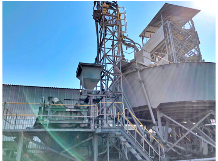
Plant View (Derrick Dewatering Screen, Hydrocyclone, and Thickener)
