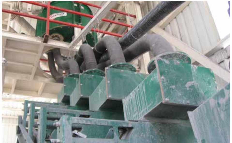
One of thirteen Derrick Stack Sizers successfully implemented at Esan Eczacibasi's lead and zinc operations at Balya, Turkey
