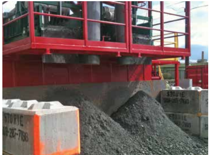
Derrick FLC 2000 shaker discharge
