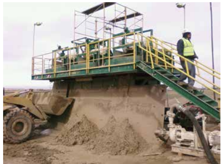
Derrick Modular Slurry Separation Plant in operation
