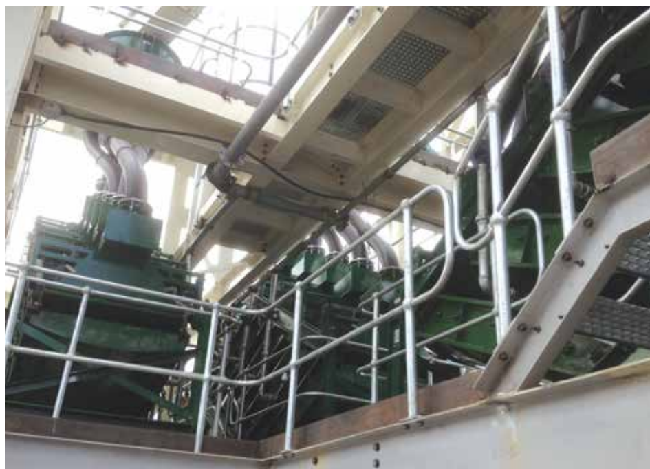
5-Deck Stack Sizers installed in early 2012
